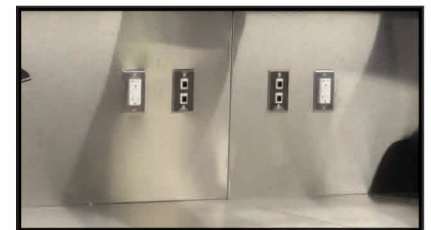
Electrical Duplex & Data Cut-Outs
